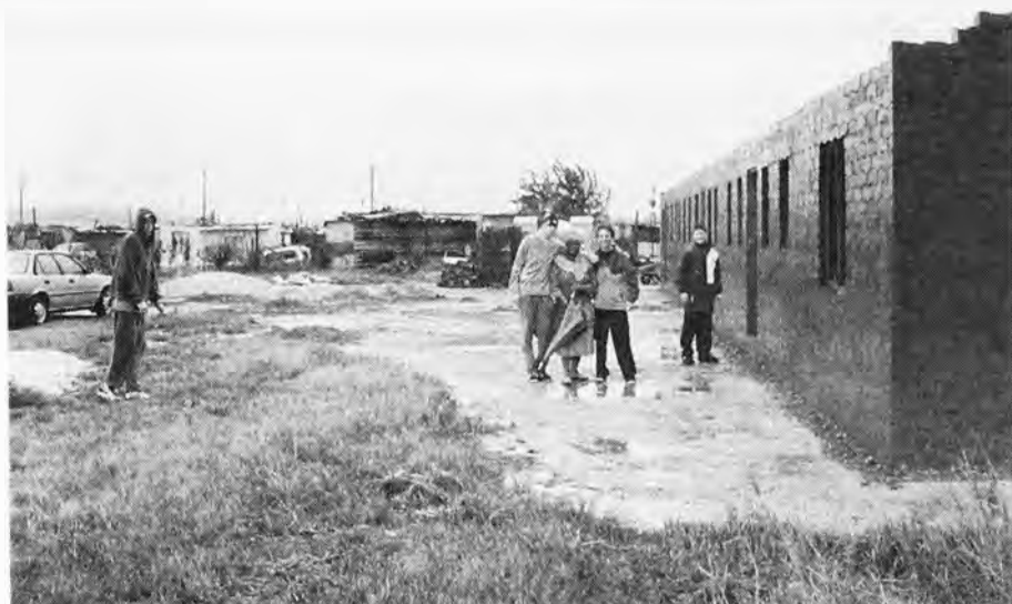
In pouring rain, women from the Catholic community in Botleng, an informal settlement outside Delmas, welcomed us and showed us around. On the right is the church-cum-school which the community is building with their own hands, with bricks made by themselves
