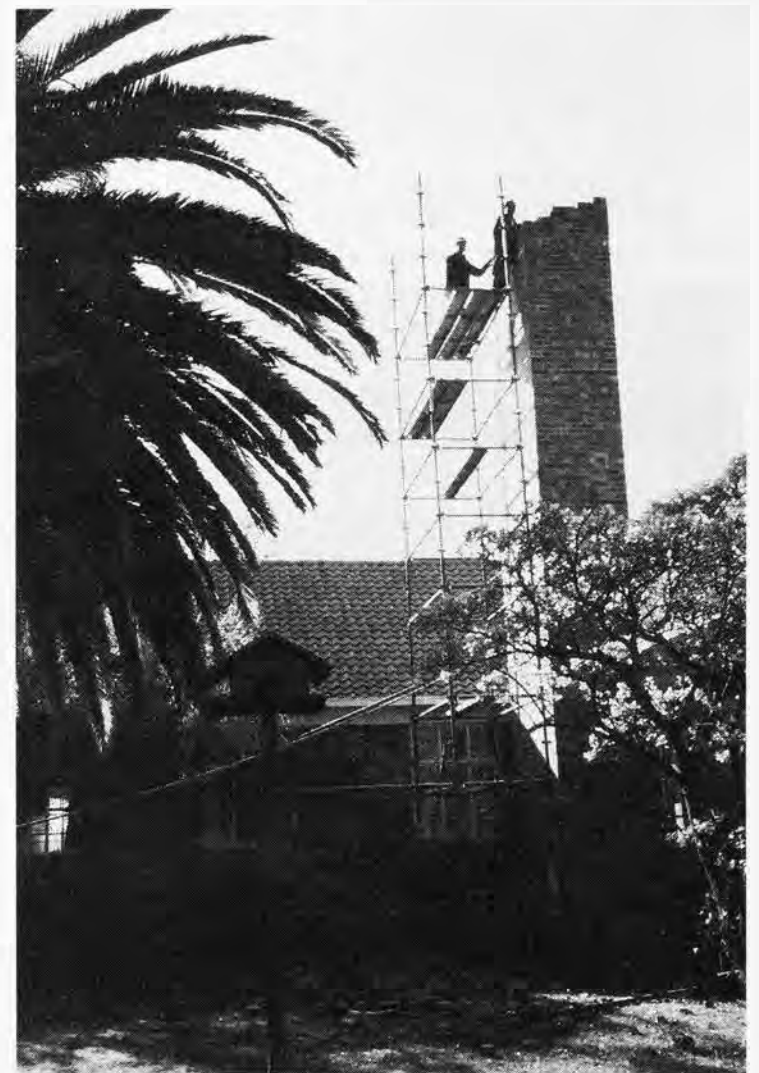
History being dismantled brick by brick as the kitchen chimney (it was once the kitchen of the boarders’ refectory) is demolished to make way for new classrooms and offices. “Development Plan 2000” has begun!
